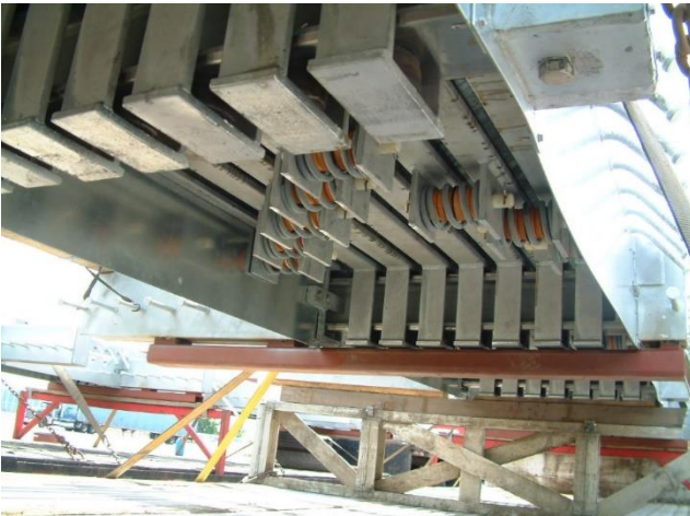
Figure 10 -- AASHTO is very clear: Welded connections are more fatigue resistant than bolted connections.
